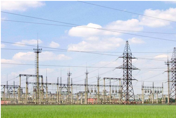
Building of HV (up to 750 kV and MV (6– 35 kV) substations
